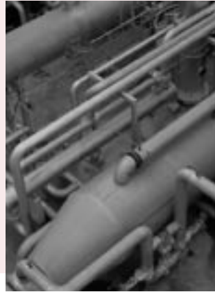
Pipelines & Pumping Stations
